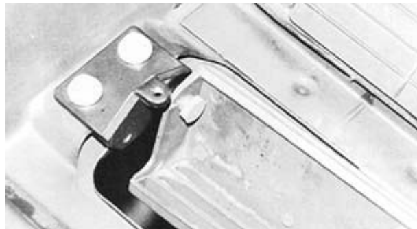
Door is aligned so it makes no contact with hood in open position.
