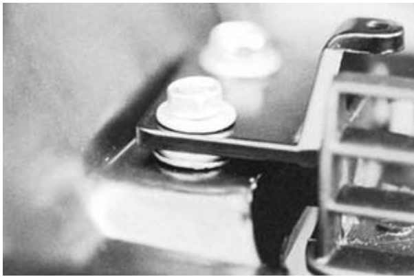
Original spacers are no longer available. Washers were used to shim flapper door where needed to level it with exterior hood surface.
